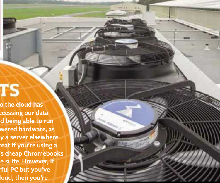
The need for cooling, a power-hungry element of most data centres, is reduced at Memset's facilities
